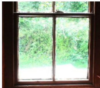
One of the old sash windows, they were in a bad way but had lasted very well for 100 years
