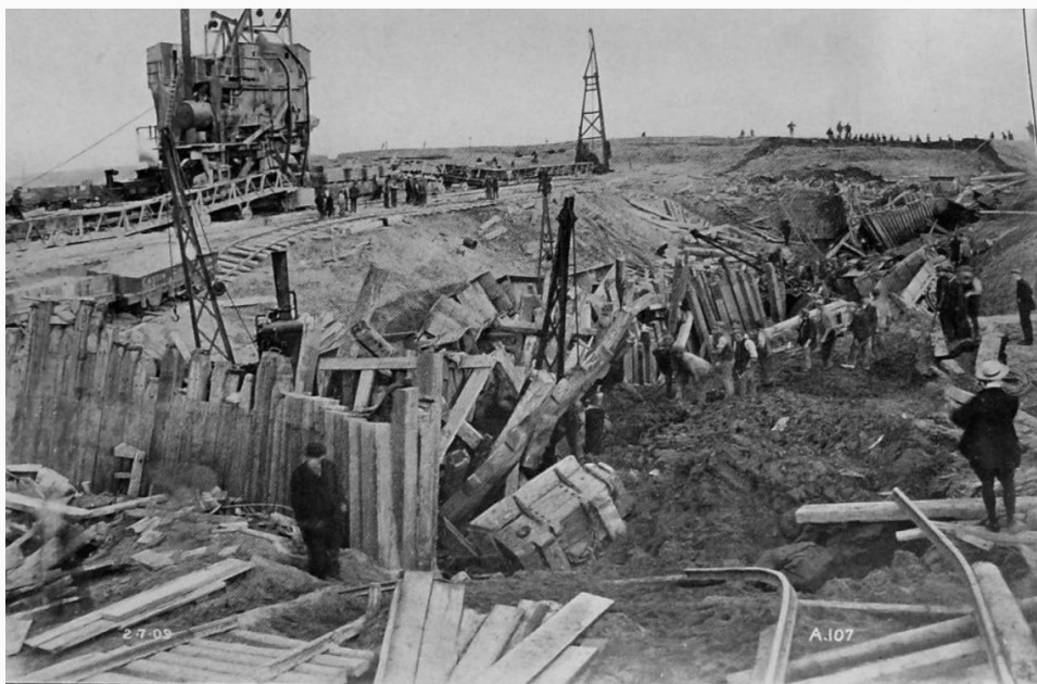
THE COLLAPSED WEST WINGWALL TRENCH, JULY 2ND, 1909, LOOKING SOUTH.
