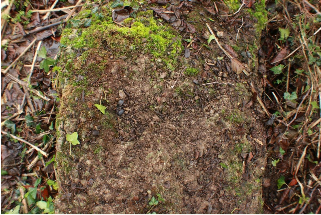
Figur 14 / Figure 14. Cymraeg: Golygfa arall o garreg sylfaen ar hyd rhediad arfaethedig y ramp, yn dangos cysondeb deunydd a lleoliad. English: Further view of foundation stone along the proposed ramp alignment, showing consistency of material and positioning.
