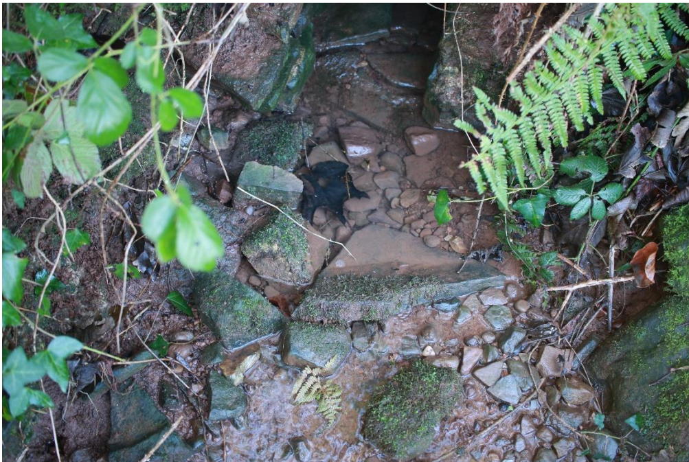
Fig 7/8 (8) Shows a 9" boxed culvert/ drain, it's position suggests possible drainage for utility buildings. Coordinates: 51.568, -3.10809
