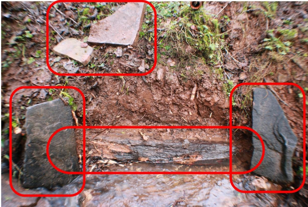
Fig 27 Showing the exercise channel edge's, approx 10/11 m width. Including timber beam in situ and possible culvert tiles/slabs. Also showing it depository position terminal to drainage waterway. Coordinates: 51.56605, -3.11533
