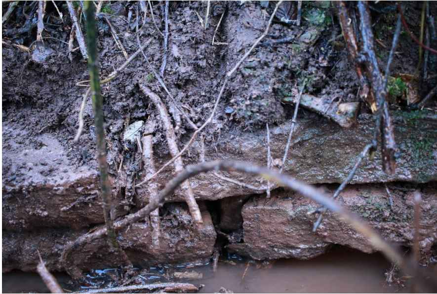
Fig 2/3 (3) Showing evidence of a possible small bridge structure that lays directly below the amphitheatre road. Coordinates: 51.56917, -3.10962
