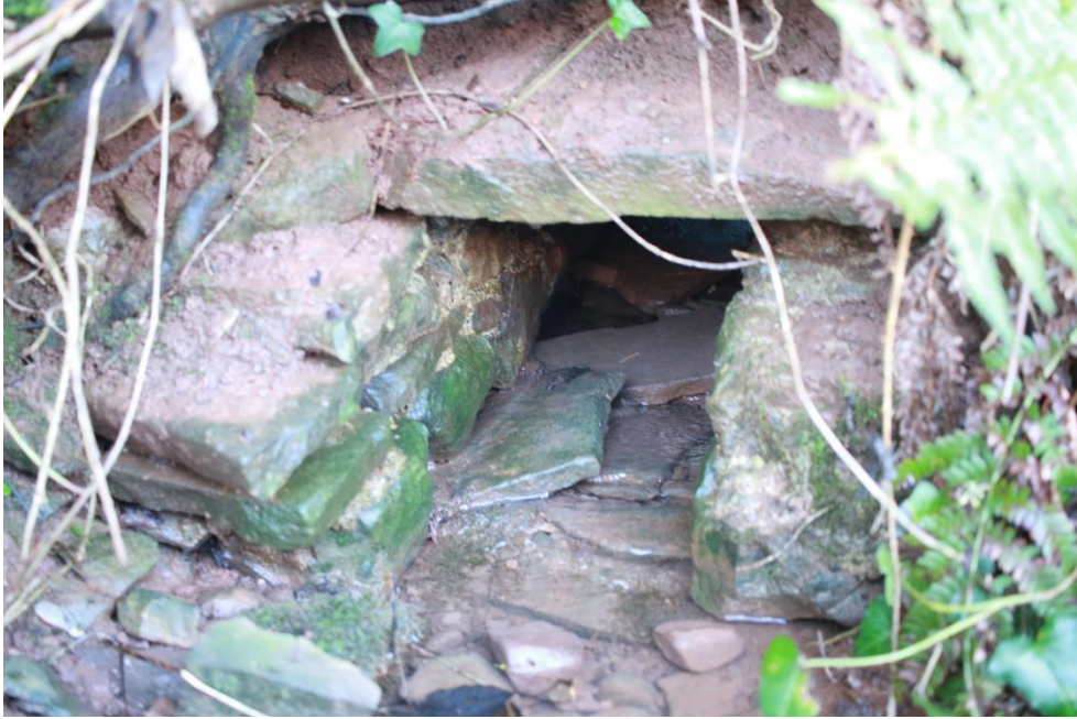
Fig 7/8 (7) Shows a 9" boxed culvert/ drain, it's position suggests possible drainage for utility buildings. Coordinates: 51.568, -3.10809
