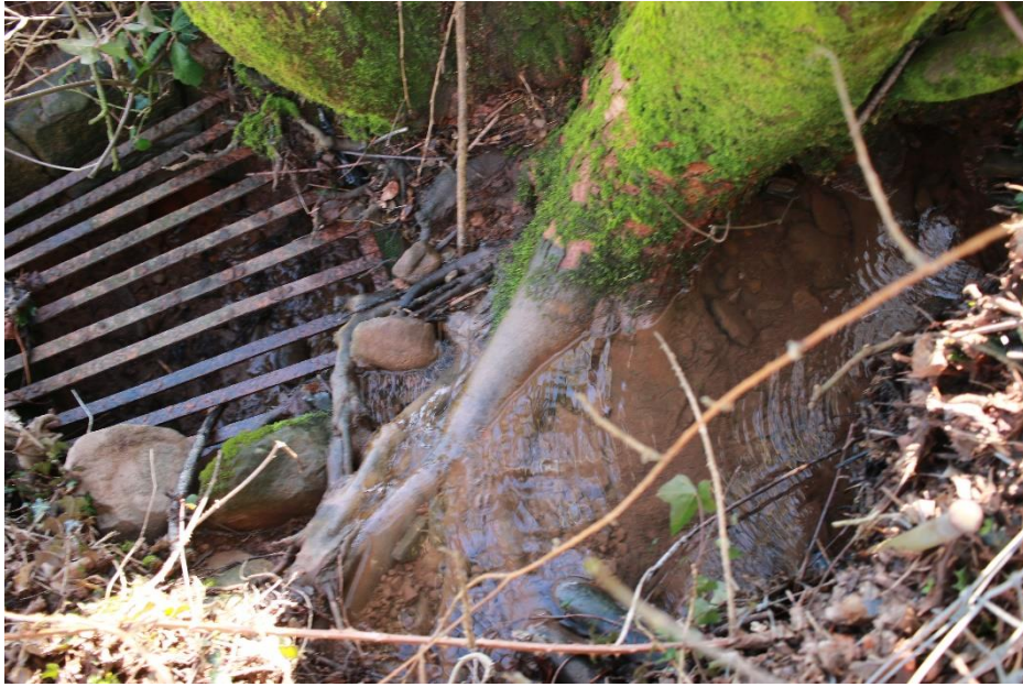
Fig 4/5 (5) Showing the grided drain sump and rounded culvert terminal the rounded terminal head down from the SW (possibly the main drain run). The defence grided sumps position is approx 45 m from centre of perimeter wall. Coordinates: 51.568, -3.10809
