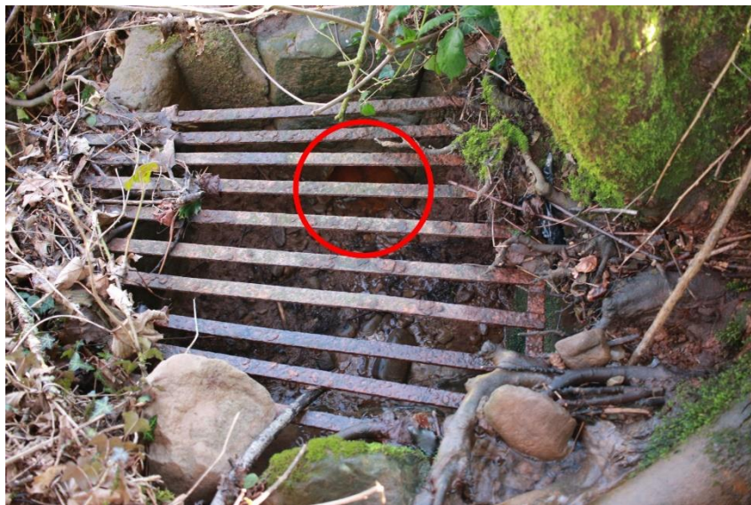
Fig 4/5 (4) Showing the gridded drain sump and rounded culvert terminal the rounded terminal head down from the SW ( possibly the main drain run). The defence gridded sumps position is approx 45 m from centre of perimeter wall. Coordinates: 51.568, -3.10809
