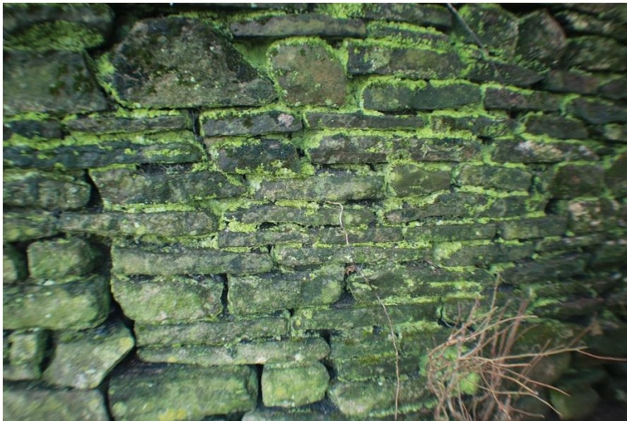
Fig 11/12 (12) Showing a buttress close to the culvert supply run. It shows signs of possible Roman stone reused. Coordinates: 51.57104, -3.11141
