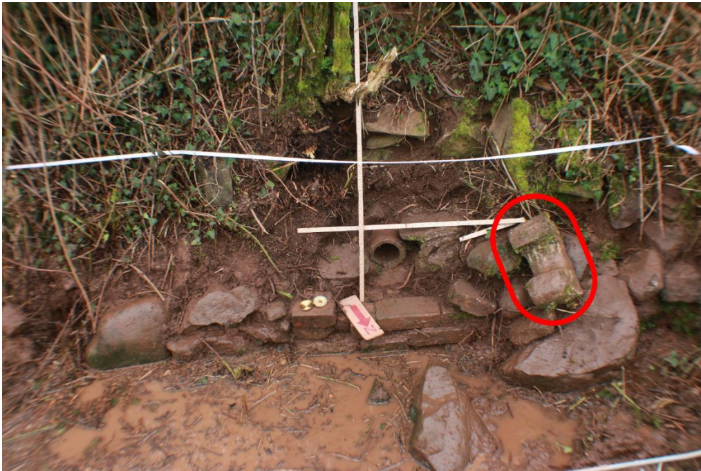
Figure 24: Masonry remains in waterway
