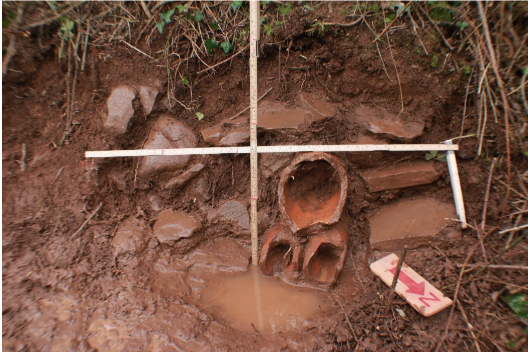
Figure 8: Triple ceramic pipe drainage terminal exiting the waterway bank with measurement scale.
