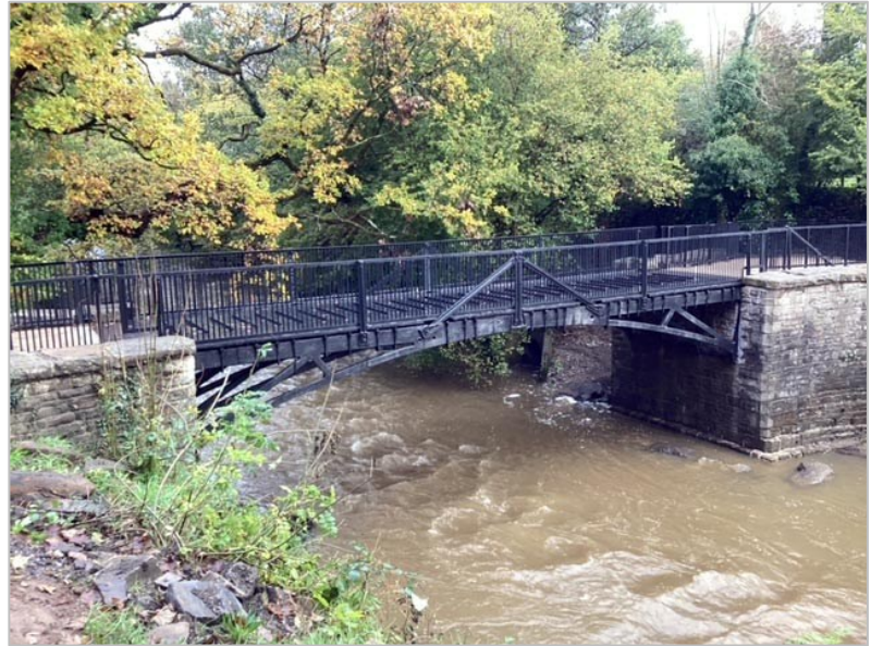
The bridge after the repairs had been completed. The handrails are a new feature.
