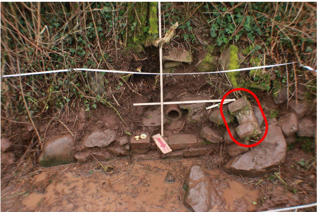
Figure 24: Masonry remains in waterway
