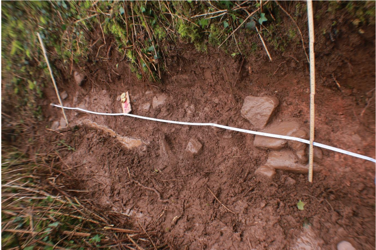
Figure 30: Detail of the road edge in Trench 7, highlighting the transition from compact surface to softer adjacent material, indicating lateral runoff or drainage.
