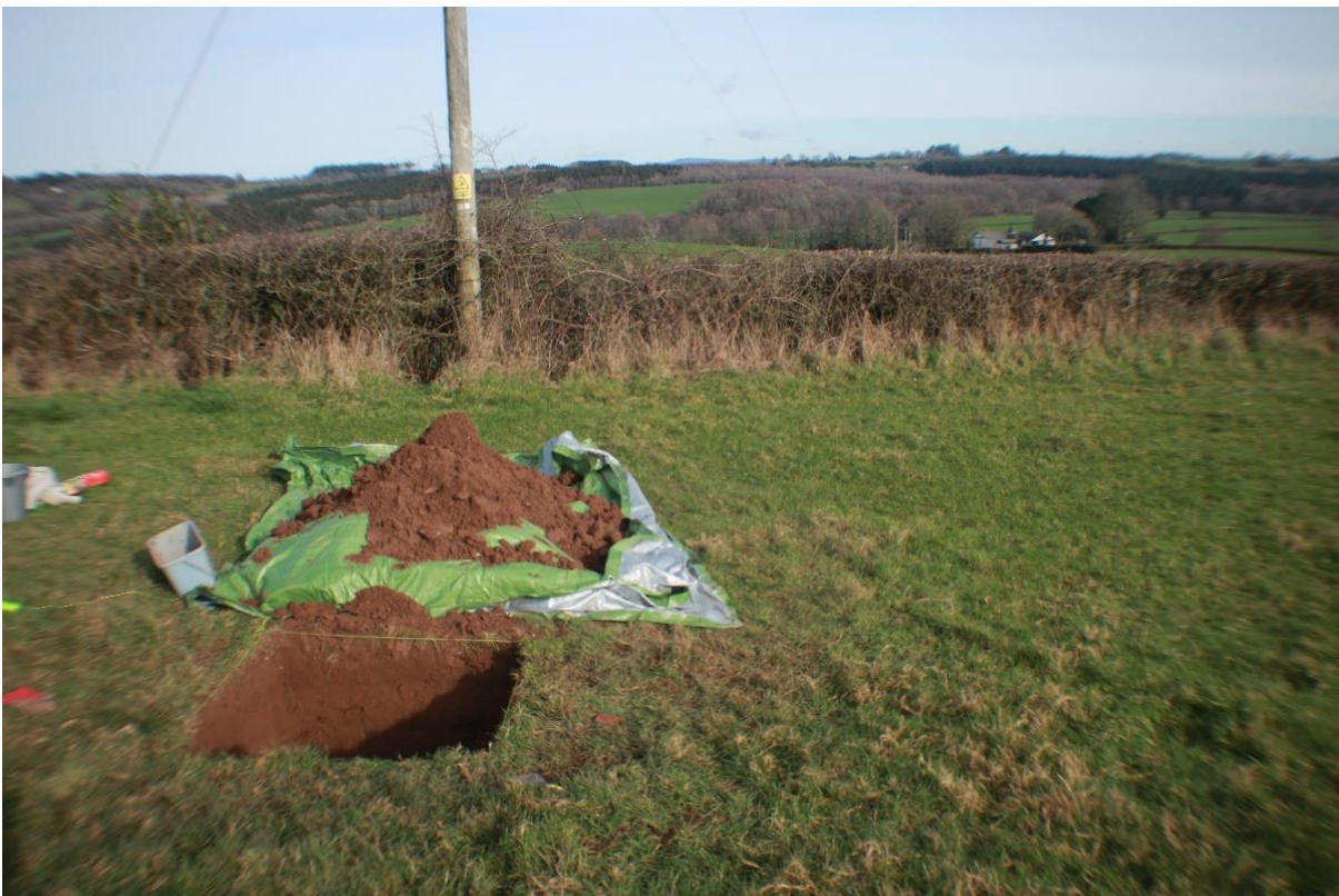
Figure 2: Location of Trench 1 positioned to investigate the predicted pipeline, roadside edge and bathhouse foundations.
