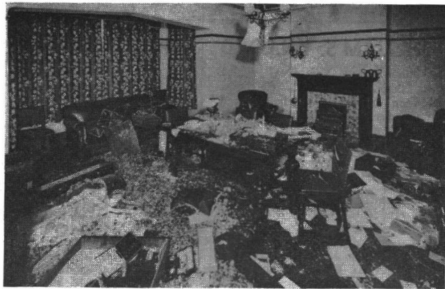
The damage caused to a room of Hillstone Grange, Stanley Road, Hoylake
