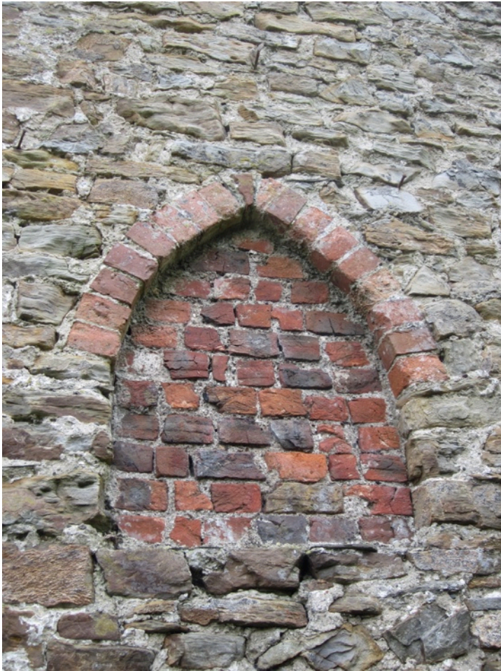
One of the high windows, showing the brick arch and the later brick infill. This window has no window sill.
